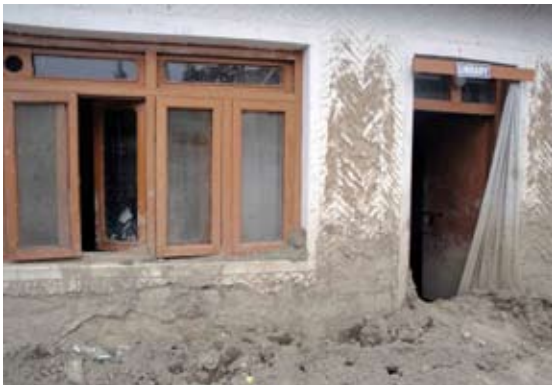
Library building before repairs.
